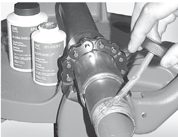
Figure 20: Application of UL listed electrically conductive corrosion protection compound on field-cut threads.
