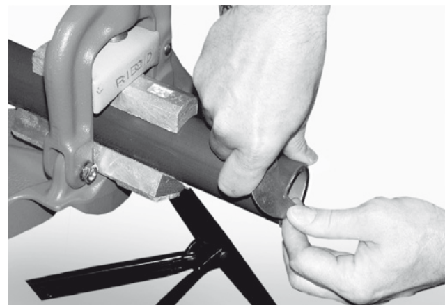
Figure 16: Utility knife used to apply "pencil-cuts" to PVC coating to allow the conduit easier entrance into the cutting die.
